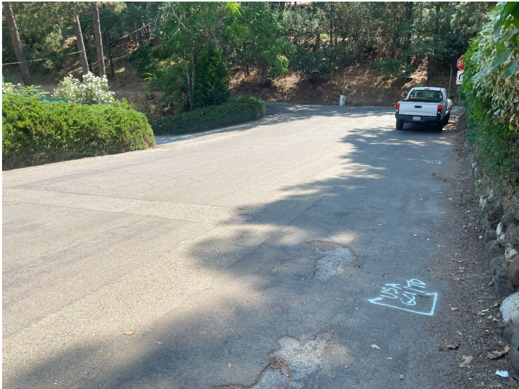
Photo No. 6 Existing pavement conditions near Boring B5 on Sherman Street (looking east)
