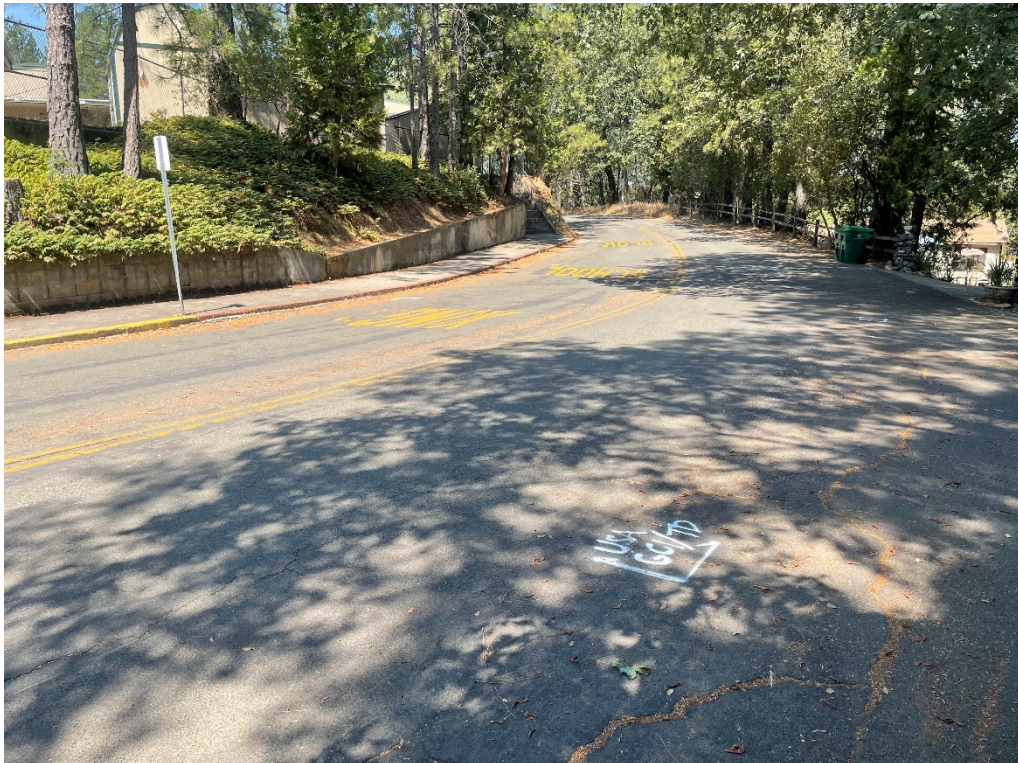
Photo No. 4 Existing pavement conditions near Boring B3 on Thompson Way (looking northwest)
