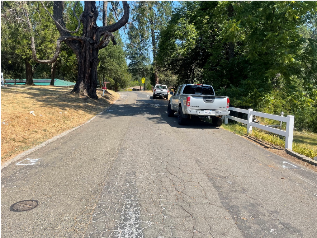
Photo No. 5 Existing pavement conditions near Boring B4 on Sheridan Street (looking north)
