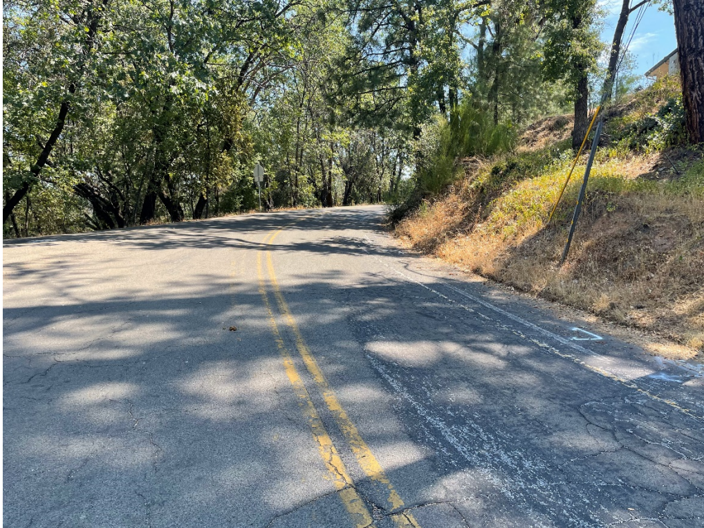
Photo No. 3 Existing pavement conditions near Boring B2 on Thompson Way (looking northeast)
