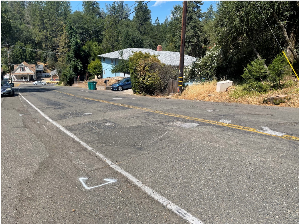
Photo No. 1 Existing pavement conditions near Boring B1 on Thompson Way (looking southeast)
